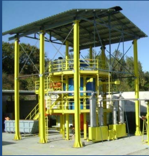
Gasification and Gas Cooling
